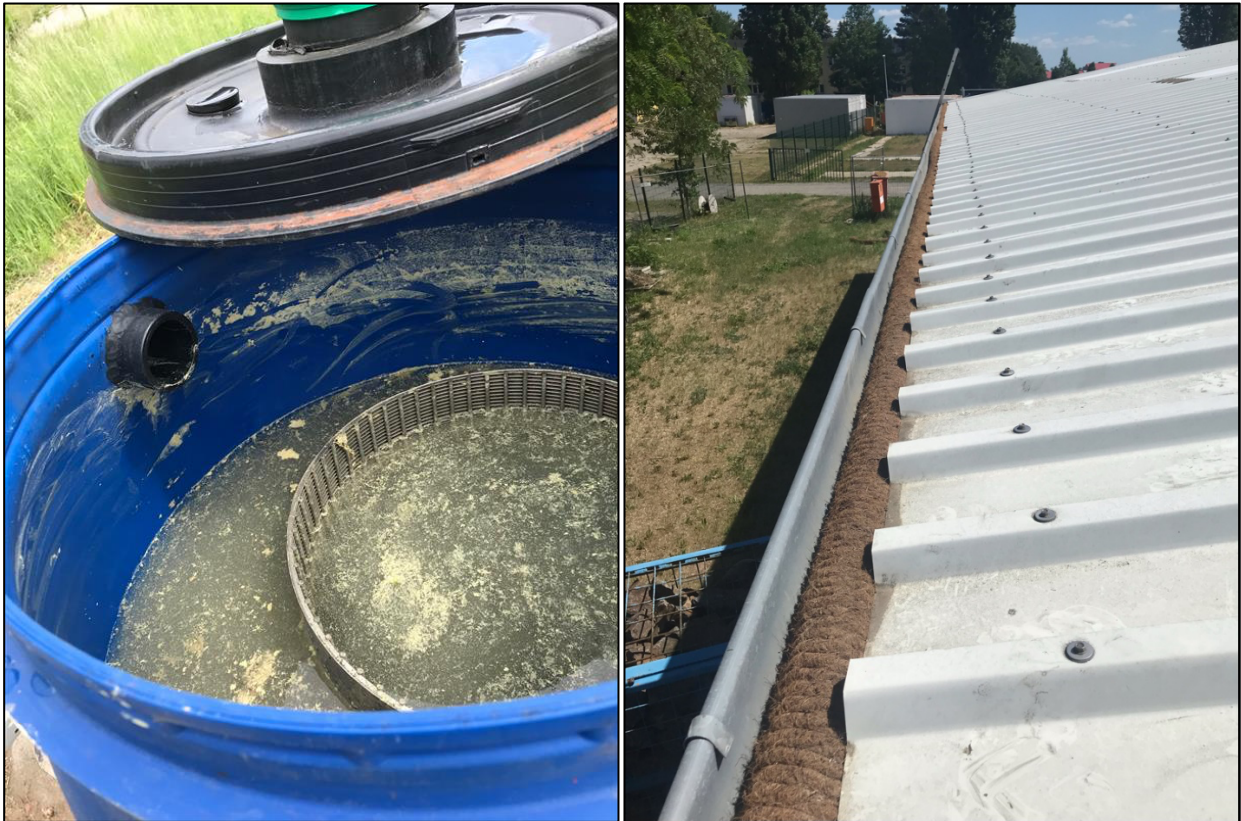
Figure 4 clogged treatment unit in June 2022 (left), coconut fiber in the gutter (right)
